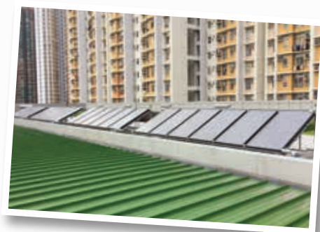
• Solar panels at Sports Centre, Community Hall and District Library Complex in Shatin
